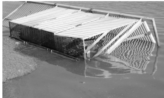
Pumps and a tidal gate on the levee east of Shorebird Marsh control tidal and stormwater flow into the marsh. High tides overwhelming this structure are a portent of impacts from rising seas to come.
